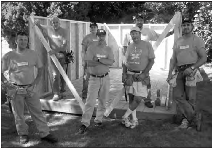
The Home Depot donated a badly needed storage shed and provided a great group of volunteers to assemble it in our backyard! The Depot Crew flanks Child and Family Services Information Technology Manager John Bassett, center.
